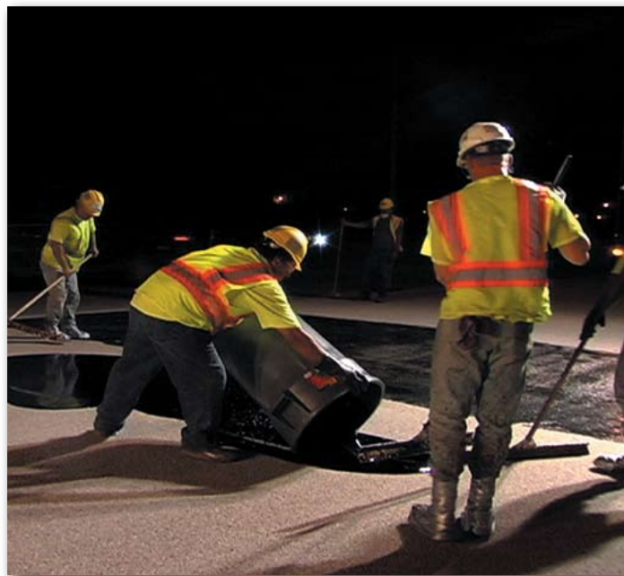
Wildcat crews lay Unitex epoxy at night to avoid disturbing traffic on Kansas' I-135 expressway.
