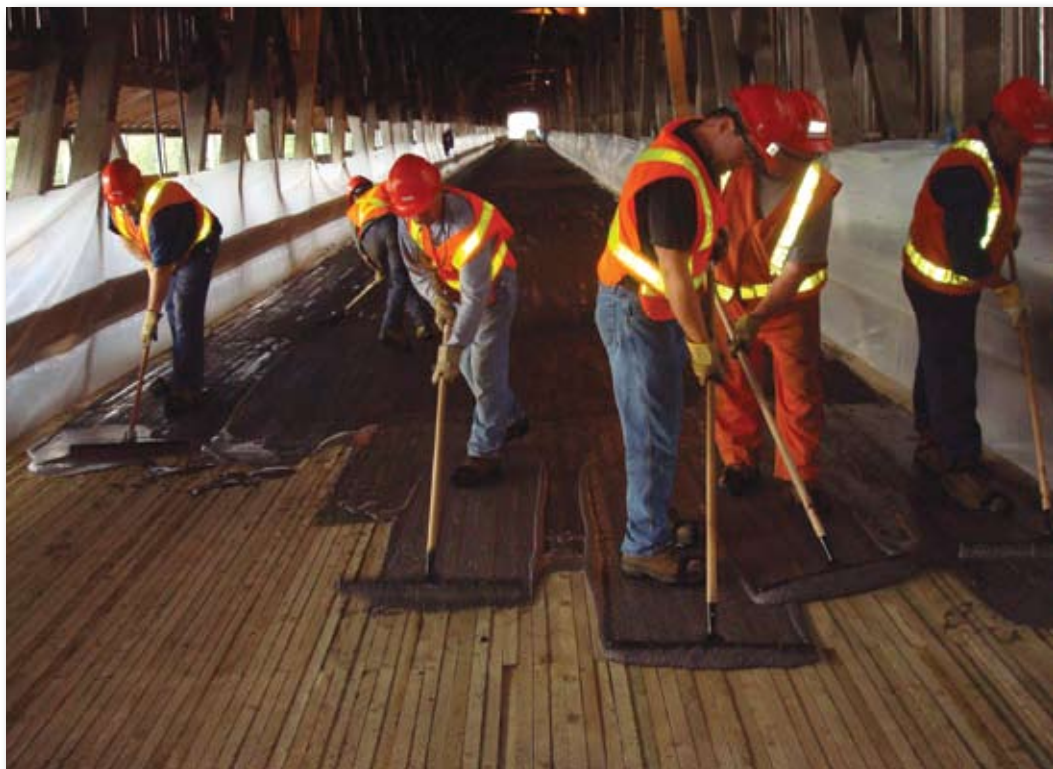
Workers spread Unitex Pro-Poxy Type III DOT epoxy to the wood deck of the world's longest covered bridge in Hartland, New Brunswick, Canada. The epoxy adds less weight than resurfacing with asphalt, which had been done previously. The overlay will extend the bridge deck's life, and make it smoother and more skid resistant.
